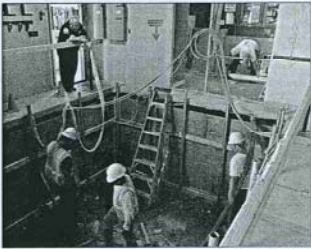
Dallas Fire Chief Bill Hahn (top, left) watches as workers pump cement into a form around what will be a new elevator shaft and support tower for the fire station.
